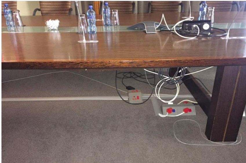
Figure 5: Existing over carpet cabling
