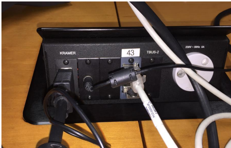
Figure 14: Existing flip top box
