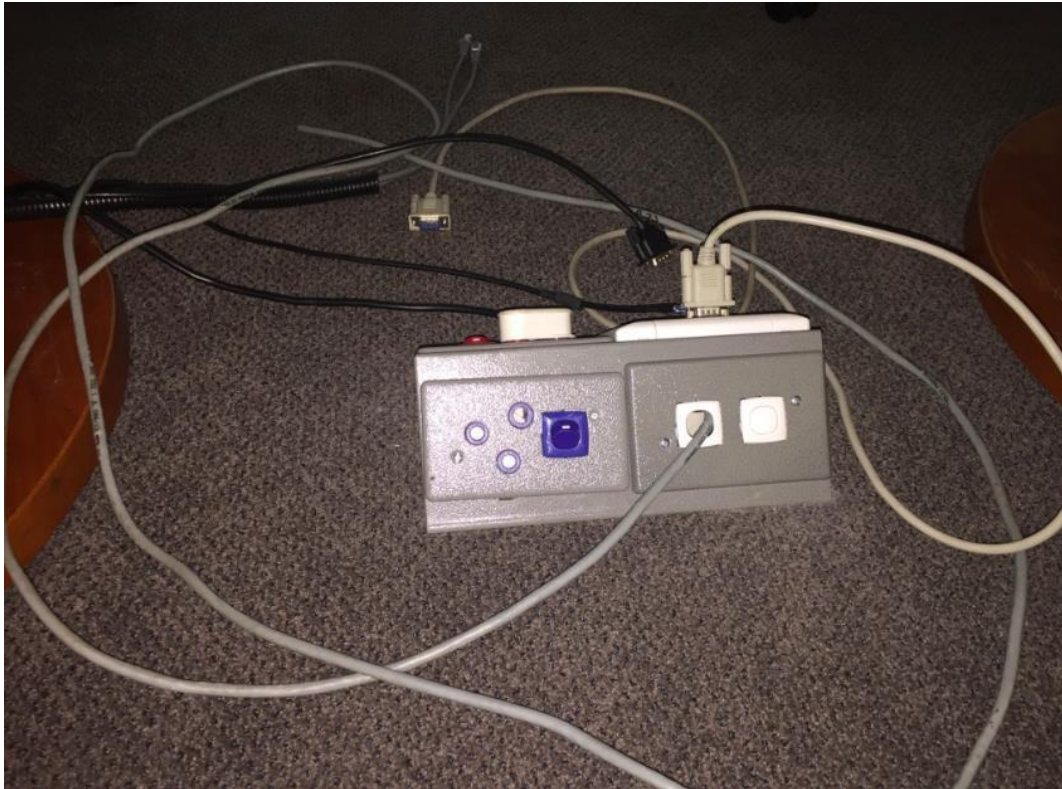
Figure 9: Current under floor trunking PEO
