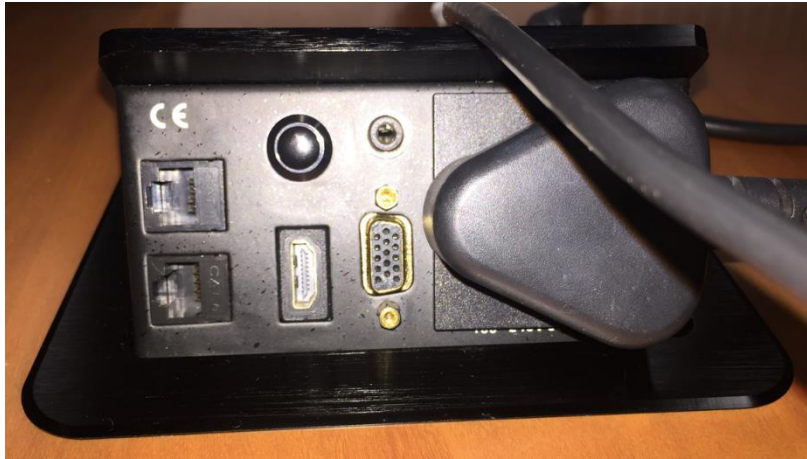
Figure 11: Existing flip top box
