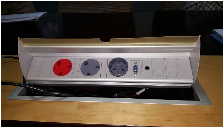
Figure 28: Existing Flip top box
